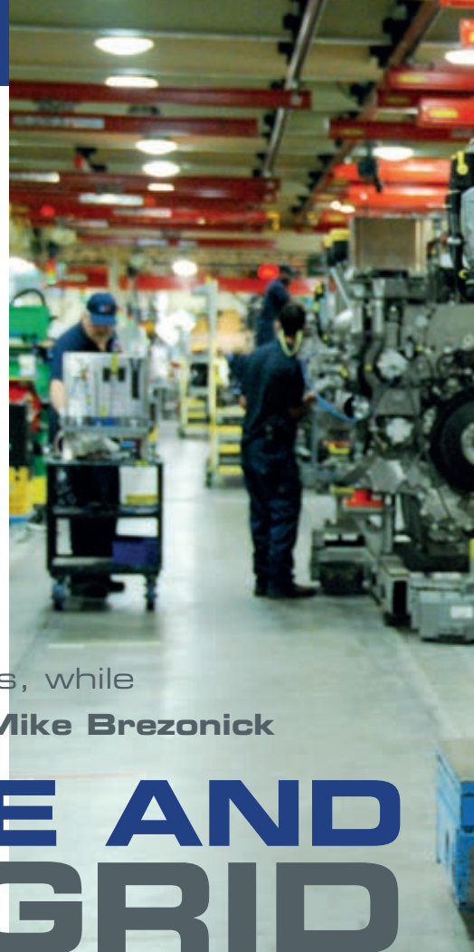
Rolls-Royce has installed a microgrid at its Aiken facility with a solar array, a Series 4000 gen-set and an mtu Energy Pack with 1 MWh lithium-ion batteries.
